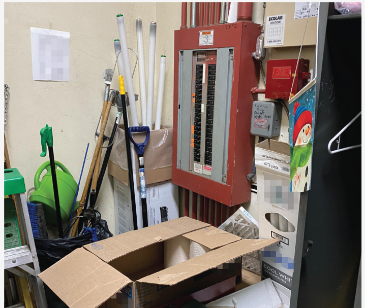
Figure 8. Blocked Electrical Panel
