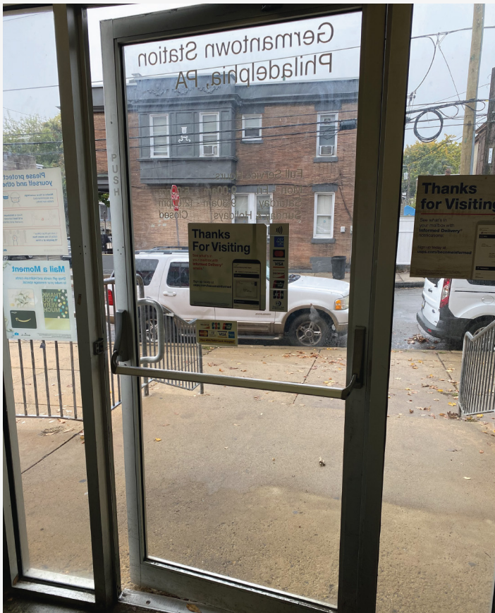
Figure 3. Entrance Door Does Not Close Properly
