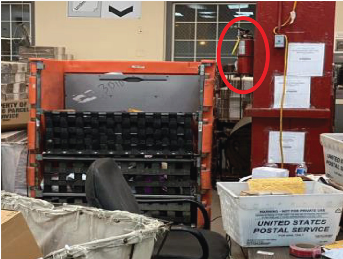
Figure 6. Blocked Fire Extinguisher
