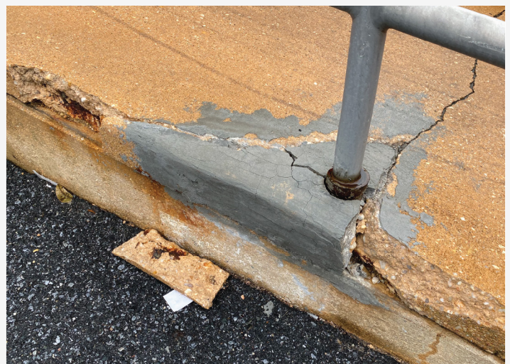
Figure 9. Damaged Ramp Railing and Broken Concrete at Rear Dock Areas
