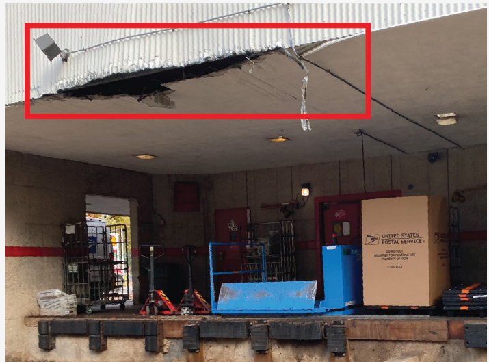
Figure 5. Large Opening in Roof Above Dock
