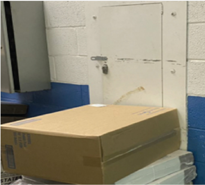
Figure 10. Blocked Electrical Panel
