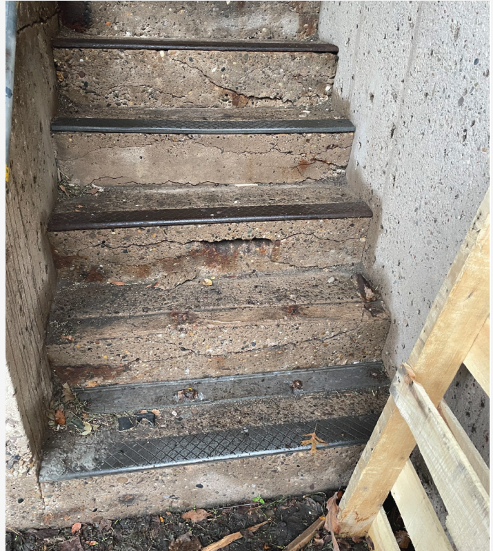
Figure 4. Damaged Dock Staircase with Multiple Tripping Hazards
