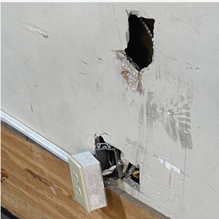
Figure 7. Electrical Outlet Not Securely Mounted and Damaged Walls
